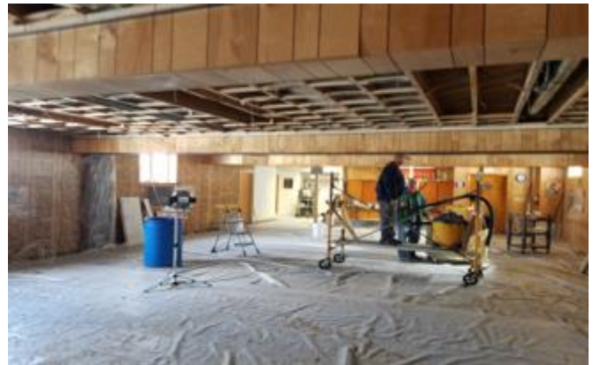
Thanks to Dale Klitz, Carl Grunewald, Ron & Donna Wuske for the installation of the new lights at Zion
